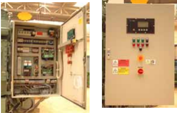
16DE CONTROL CENTER
