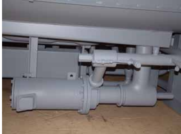
VIEW OF TYPICAL HERMETIC PUMP/MOTOR ASSEMBLIES
